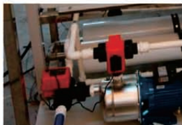
○ 海水淡化设备 Seawater desalination equipment
