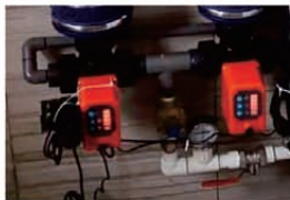
○ 反渗透设备 Reverse osmosis equipment
