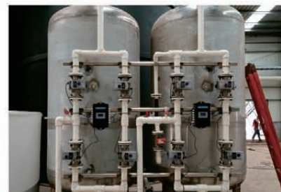
○ 造纸厂75吨锅炉用水 75 tons boiler water system in paper mill
